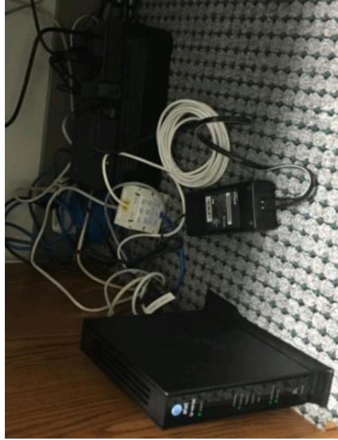
AT&T Firewall / Modem / Wireless AP DSL Line & UPS
